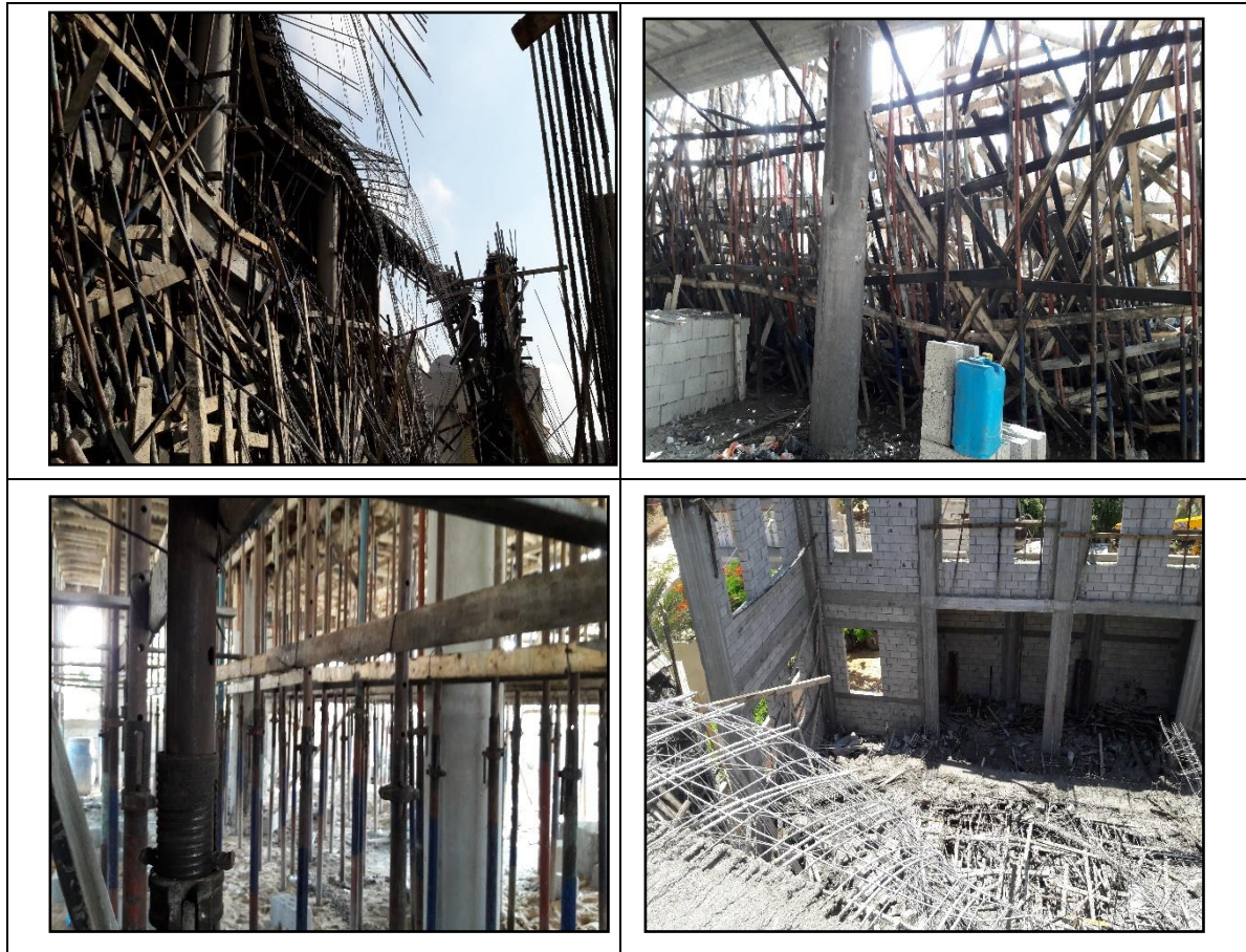
Figure 3: Photos of the failure of Abu Baker mosque.
