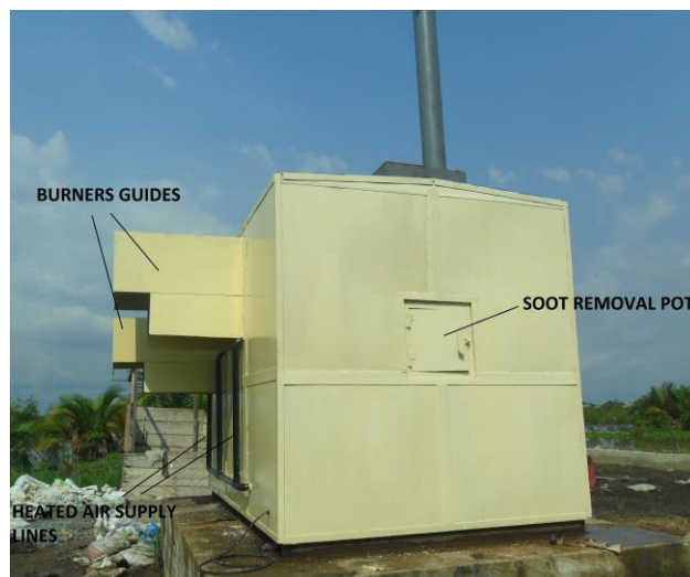
Figure 3 Pictorial view of Installed Incinerator
