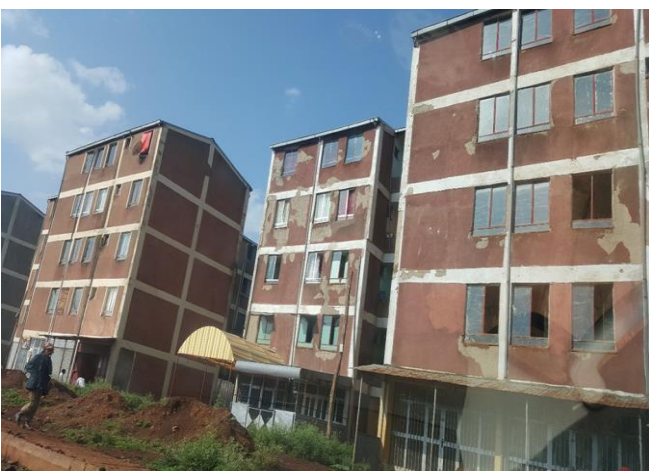
Fig 3. Peeling of paint on the wall (Saris site)
