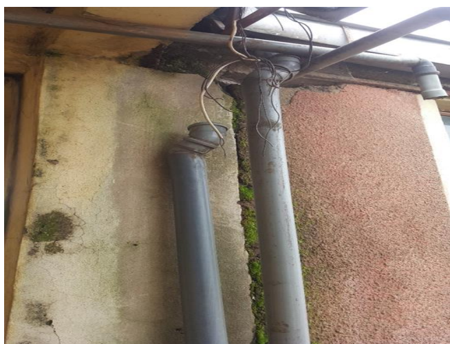
Fig 6. Mold and Fungi on the wall
