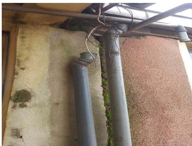
Fig 6. Mold and Fungi on the wall
