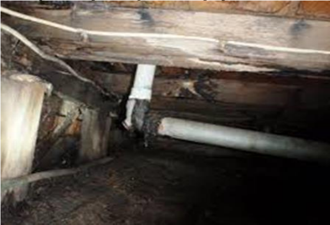
Fig 2. (b). Leaking of pipes in toilet
