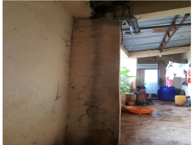
Fig 4. Cracking on the wall and Floor
