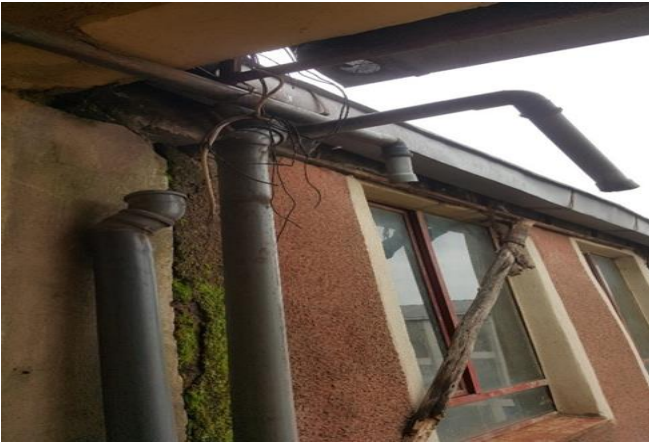
Fig 2. (a) Pipe leakage due to improper connection.
