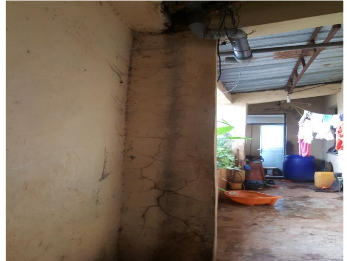
Fig 4. Cracking on the wall and Floor
