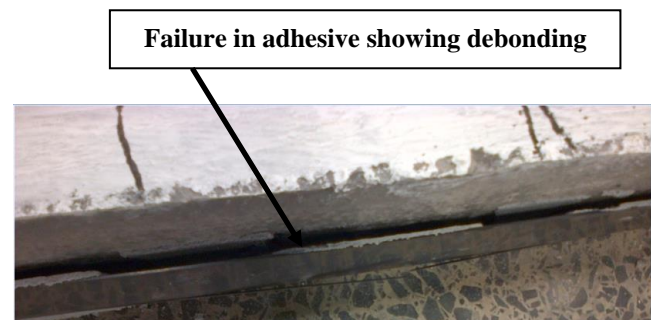
Figure 13. Intermediate crack induced debonding (b)
