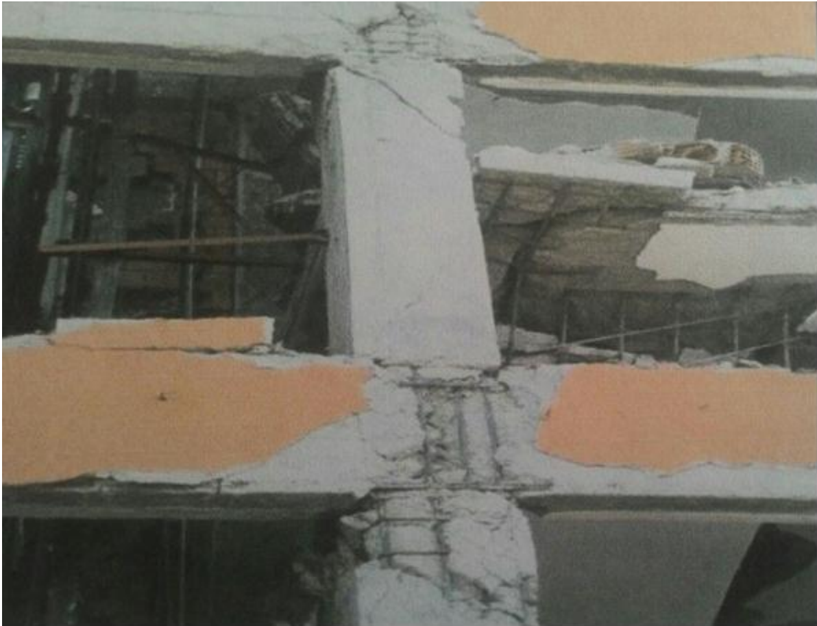
Fig. 9 Inadequate Reinforcement Detailing of Collapsed Beam Column Joint
