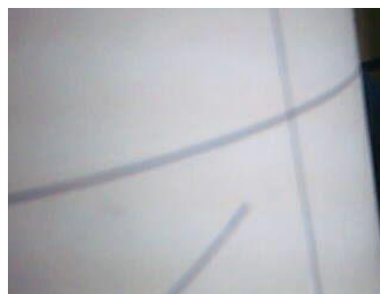
Fig.8 Tile having inclined crack
