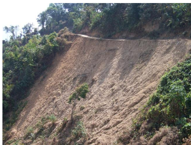
Plate 2. Road being disrupted by landslide occurred below Hnahthial College
