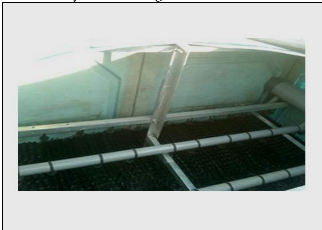
Figure 8. Water distribution system of cooling towers
