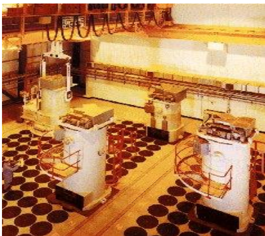
Fig: Loading silos with canisters containing vitrified HLW in the UK. Each disc on the floor covers a silo holding ten canisters
