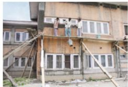
Fig. 3 One of the structures in Kashmir where Retrofitting work was in progress by making use of IS 1893-2002
