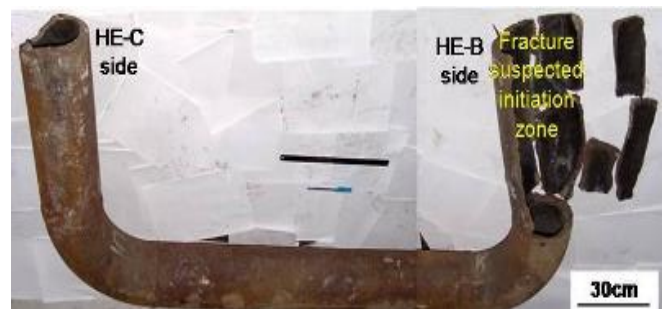
Fig. 1. General view of the fractured U-bend pipe joint connecting the heat exchanger B (HE-B) to the heat exchanger C (HE-C).
